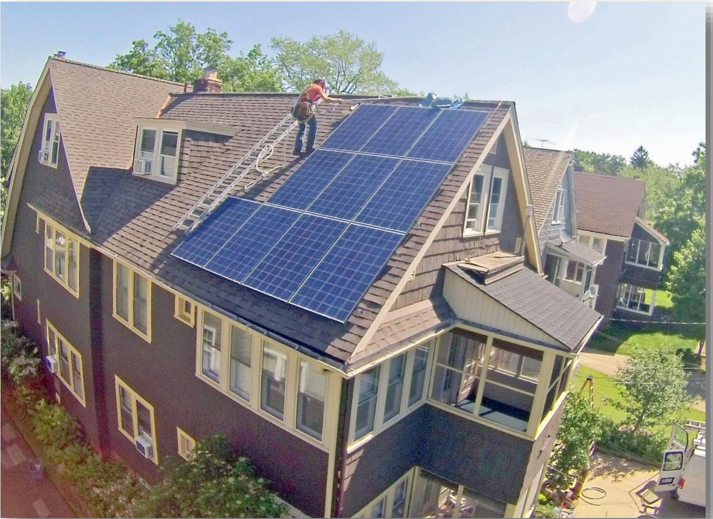
Residential solar installation in Cleveland Heights by AAT Solar. How can communities facilitate the expansion of clean power?
